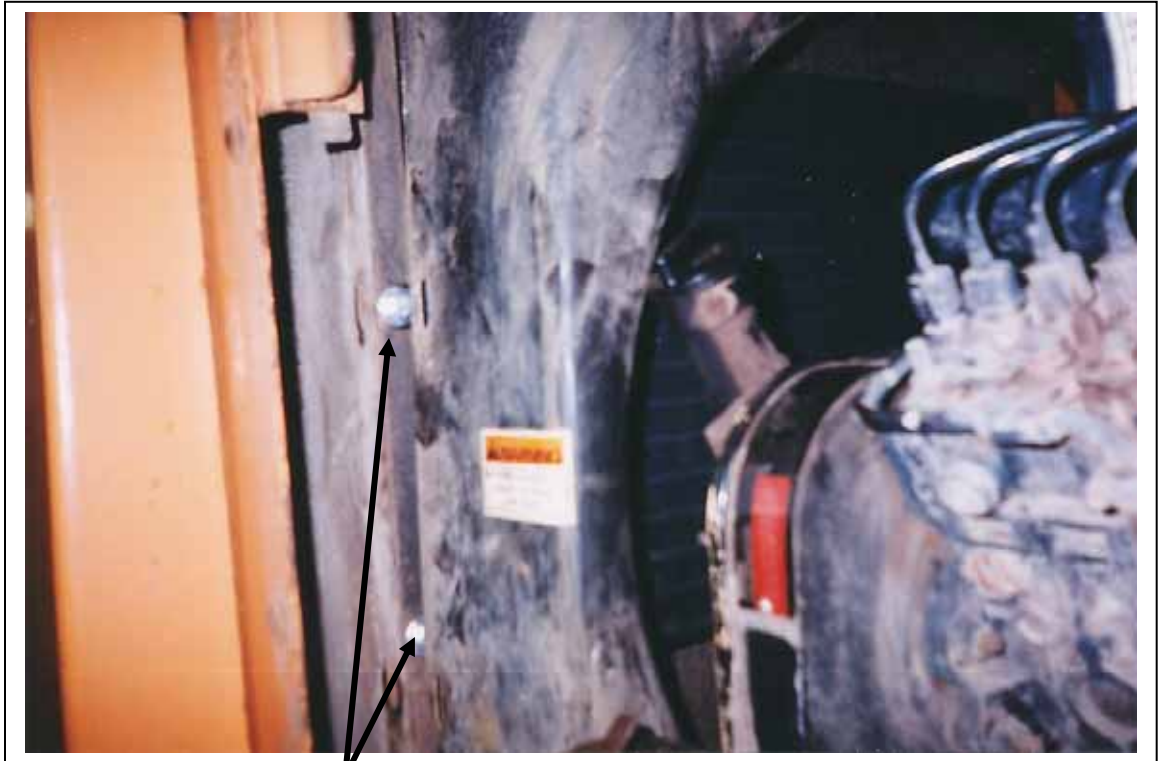
Bolts holding condenser brackets in place
