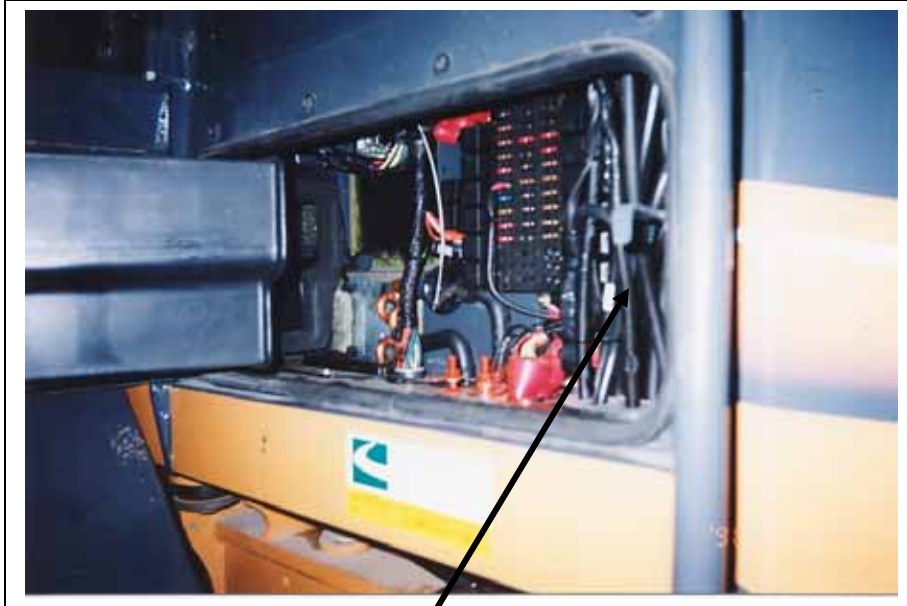
Clutch wire in electrical compartment on right of cab. Run over to the thermostat keeping clear of the filter intake cover.
